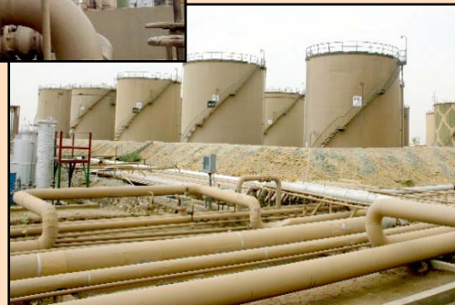
Product Storage Tanks
