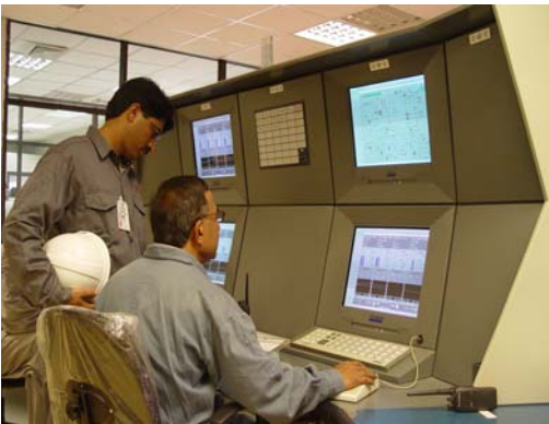
Central Control Room
