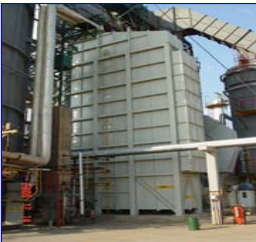
Waste Heat Recovery Unit
